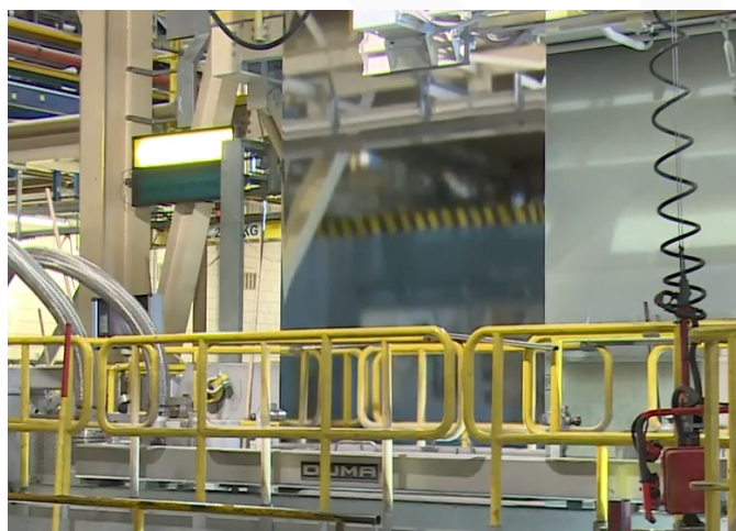
Hot Dip Galvanizing - Induction Furnace
